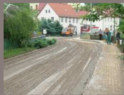
Gradual destruction due to water erosion
